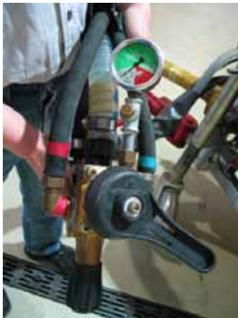
Fig.5: Manually operated control valves
